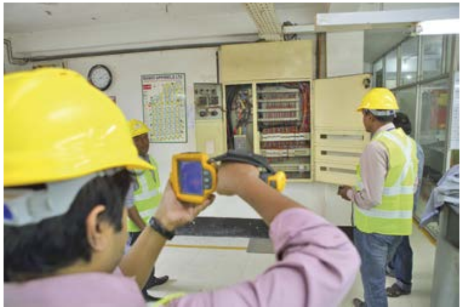
↑ Assessing an RMG factory for electrical safety. In the aftermath of the Rana Plaza collapse, all export-oriented RMG factories have undergone inspection for structural, fire and electrical safety.
